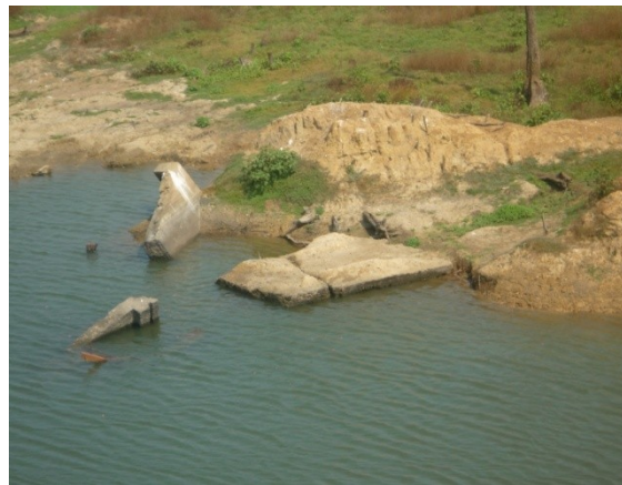
Fig 3.2 Part of the washed off sluice
