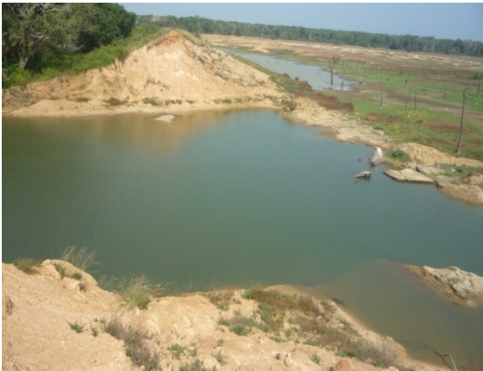
Fig 3.1 breached section of the dam
