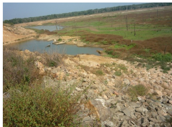
Fig 3.3 washed off section of the Rip-rap
